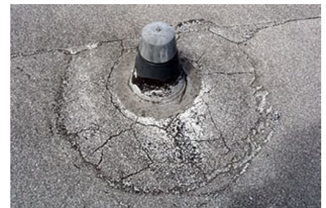
Aged and cracked coating creates an entry for water that eventually leads to more costly damage.
